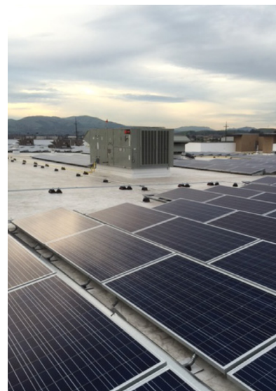
Solar panels on roof of a Nordstrom Rack store
